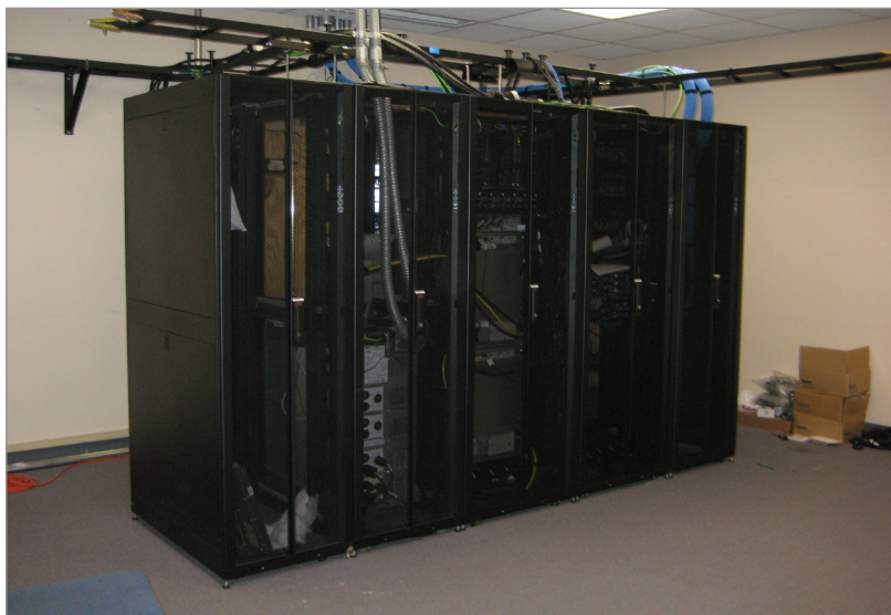
New server room at Douglas (AZ) Public Library.
